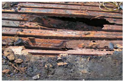
Seriously deteriorated Steel deck
