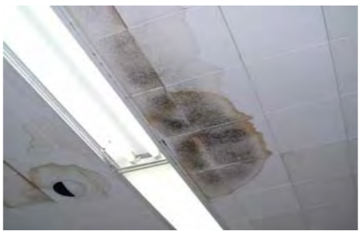
Black mold on Ceiling Tiles
