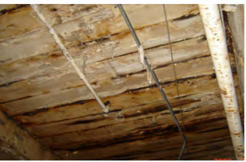
Seriously deteriorated Wood deck
